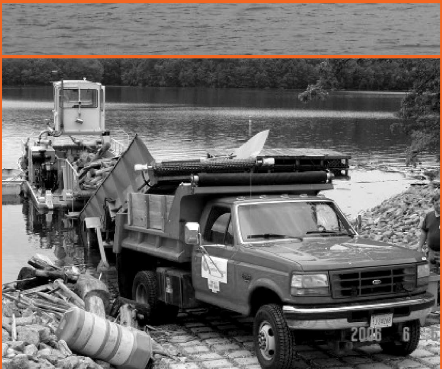
Lilli-Zoarus Rex unloading woody floating debris removed from Lake Lillinonah at the Ramp near the Shepaug Dam
